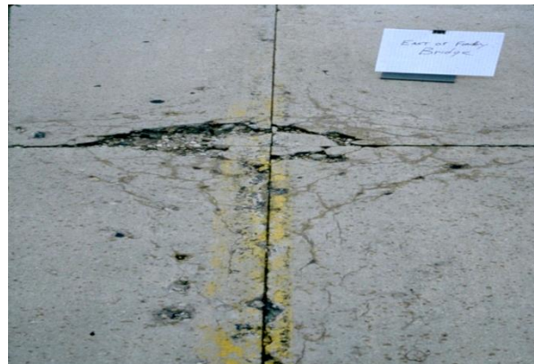
Pavement damage from D-cracking
