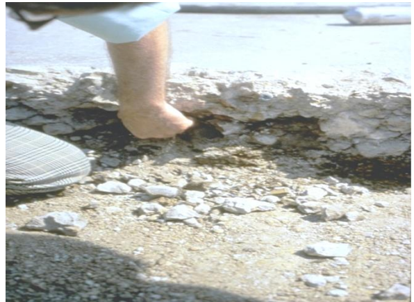
Pavement damage from D-cracking
